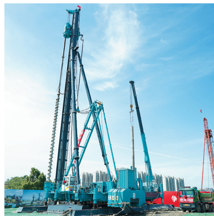
The NZEB project marks a major step toward sustainable and energy-efficient development in Jiading.
