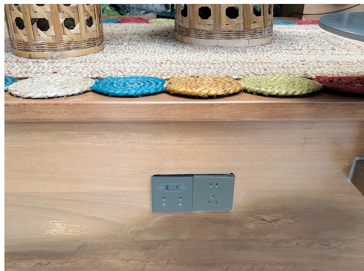
Customers can charge their phones at step-embedded sockets powered by rooftop photovoltaic panels.
