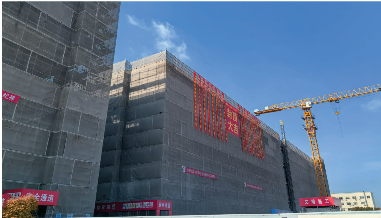
A topping-off ceremony was recently held to mark the completion of the structural framework for Phase I of Valeo's Comfort and Driving Assistance Systems Manufacturing and R&D Base in Waigang Town. — Li Pin
